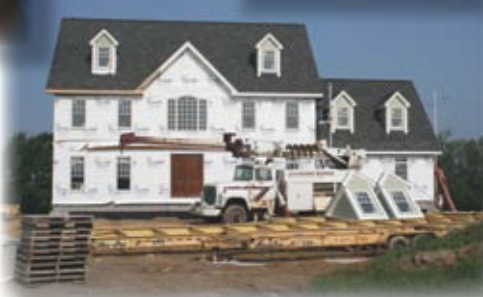
After the dormers are set to place the house finally takes shape.
